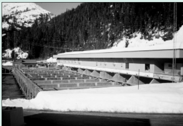
Snettisham's concrete raceways will be resurfaced and covered by steel enclosures this summer.
