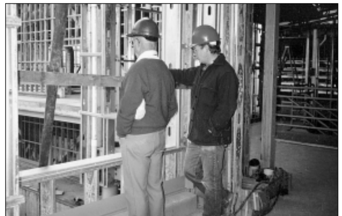
Ladd's careful scrutiny and attention to detail was essential to the construction of the Gastineau facility in 1989. In this picture he talks with Hugh Macaulay as the hatchery building is being framed in.
